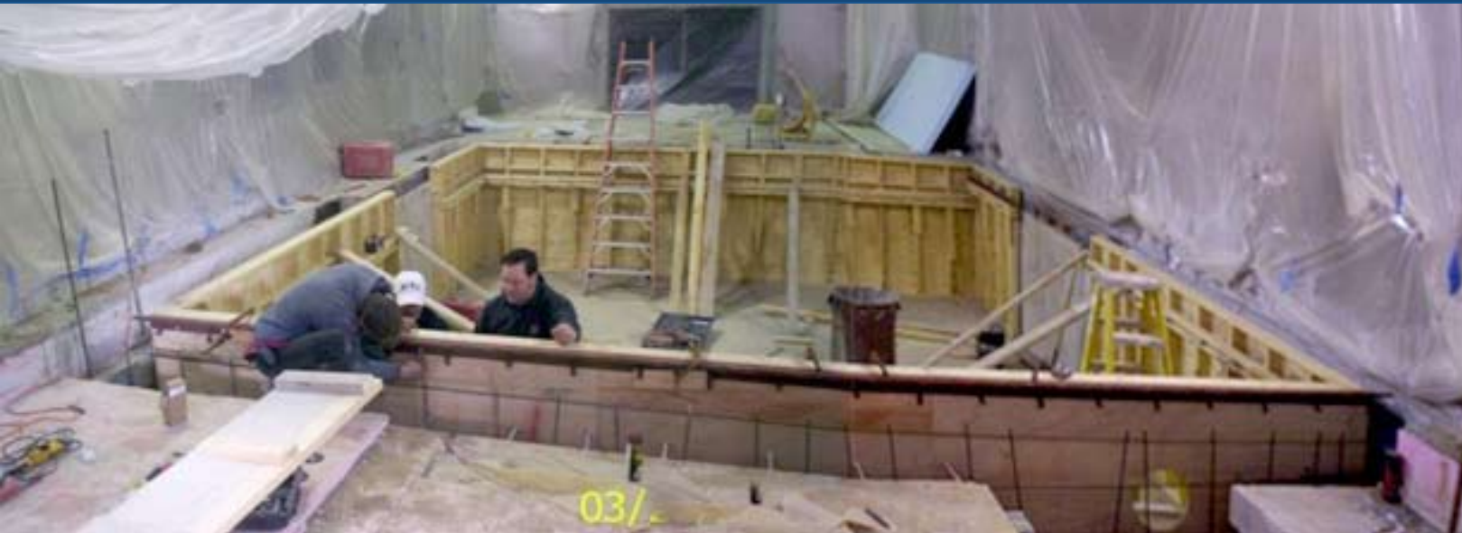
↑ Photo of new pit under construction. MAE was successful in completing the entire upgrade of this test cell in under one month by carefully planning all phases of the construction to coincide with the design and manufacture of the equipment portion of the project.
