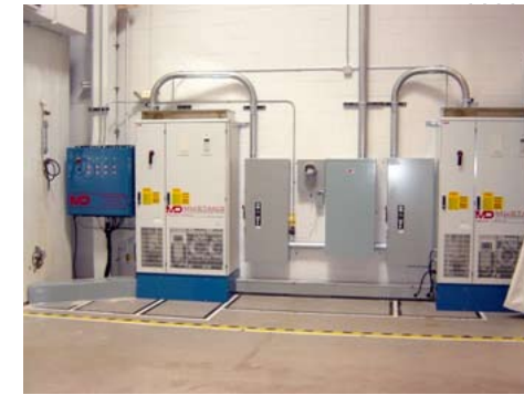
← High power control area outside of test cell door.
