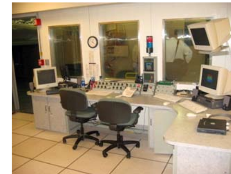
← Control room with new PC and dyne controls.
